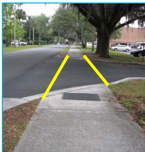
Missing Crosswalk on College Ave
