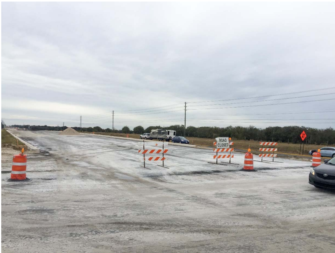
Photo 31: Northbound Lane looking South at Intersection of Superior Blvd. at Greater Lakes
